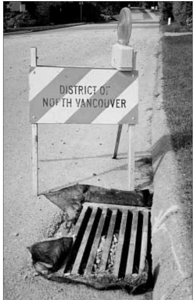
The District of North Vancouver uses stormwater grate inserts for its road works (above). Youth teams organized by Planet CPR in Washington (left) install inserts as a fundraising activity.
